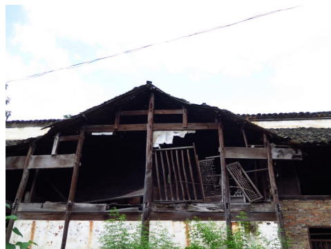
Fig. 1. Photo of damage of ancient building structure.
