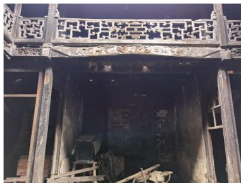
Fig. 2. Photo of damage of ancient building technique.
