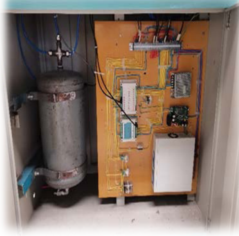
Fig. 5. The interior of the equipment.
