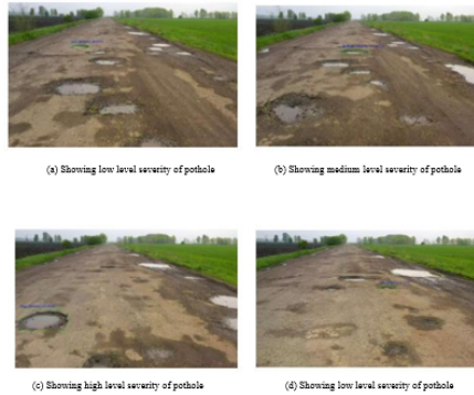
Fig. 3. Severity levels of potholes
